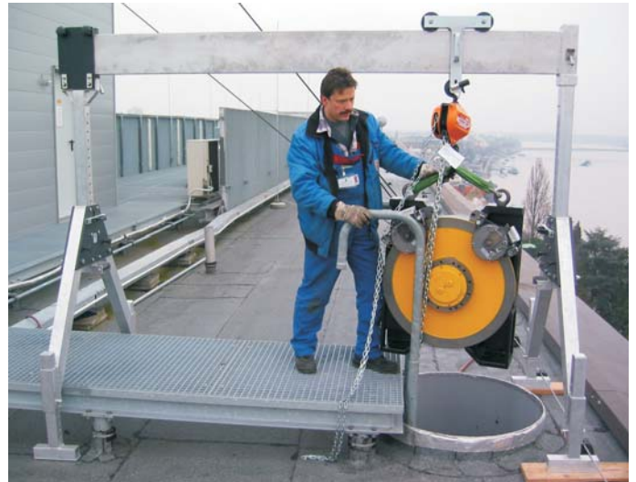
Aluminium gantry crane moving a motor
